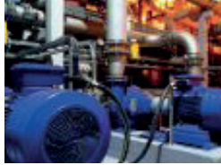
Handling Equipment & material processing
